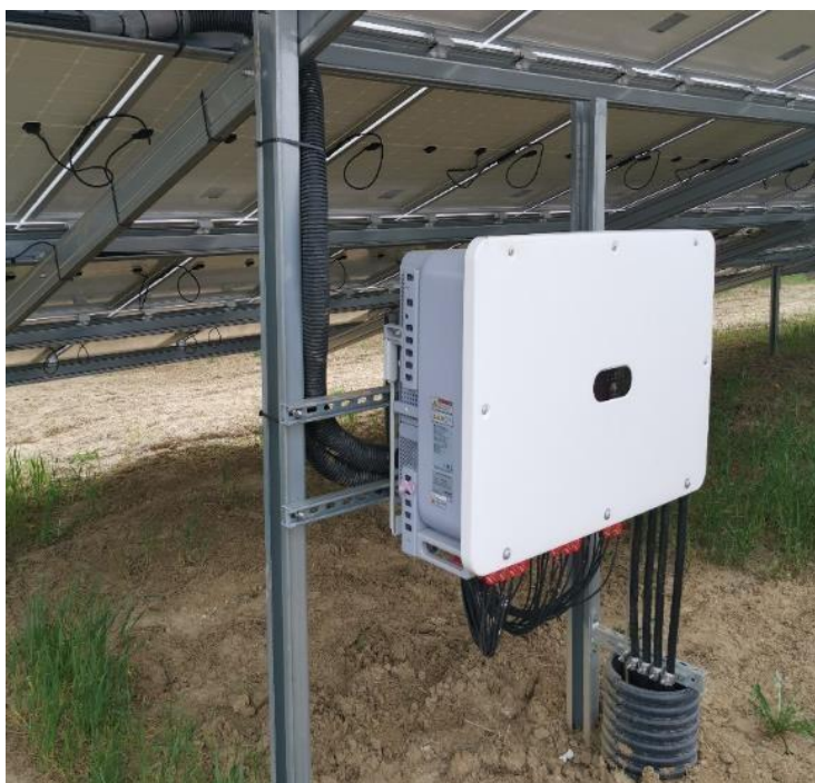
Fig. 7 – Inverter montato in campo
